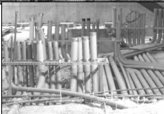
Feeder conduit for electrical room switchgear
